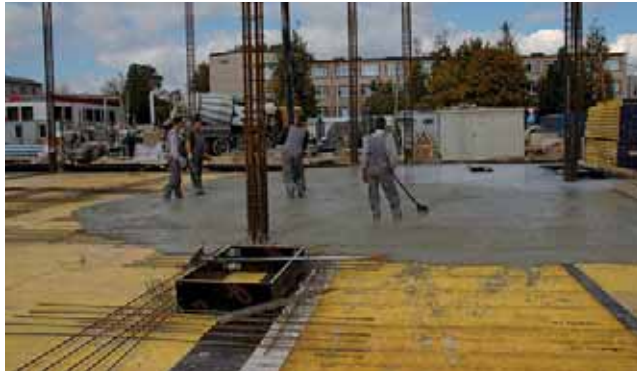
Figure 8: A 250mm TAB Slab being poured at Ditton Nams shopping mall project (Daugavspils, Latvia). APC bottom reinforcement from column to column is visible.
